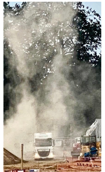
Dust storm at Chapel Field: problems for Grundisburgh residents from Hopkins building site. More on page 13.
